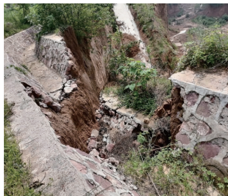
图 19 极端降雨导致截洪沟局部滑塌 [16] Fig.19 Extreme rainfall triggered partial collapse of the flood trench [16]
